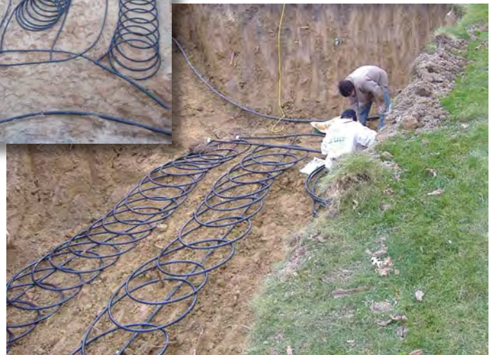
Workers at Don-Martin Heating, Cooling & Geothermal in Janesville install a vertical loop ground source heat pump system. The loops are fluid-filled polyethylene pipes that absorb heat from the ground and transfer it inside during the winter. (Photos courtesy of Don-Martin Heating, Cooling & Geothermal)
